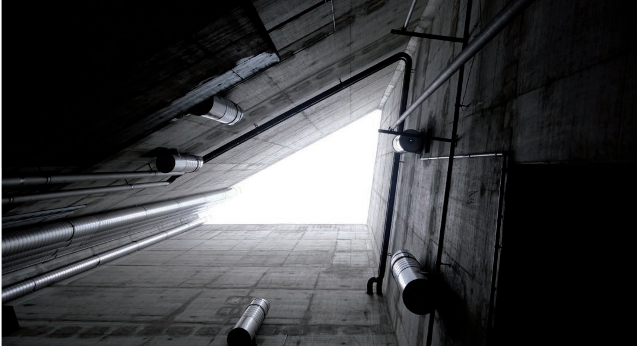
The triangular space in the middle of the parking garage, seen from the level of the waterbasins
