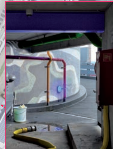
The project reveals the existing infrastructure and offers it temporary to the public.
